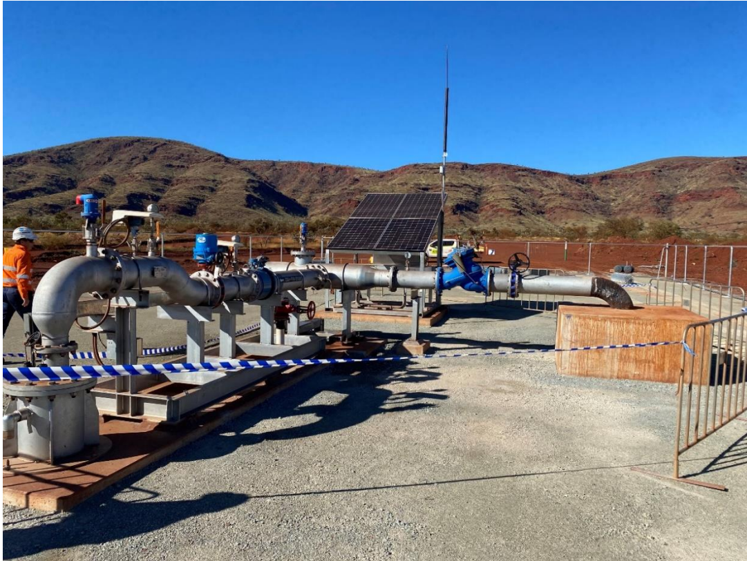
A new MAR bore at South Flank – part of the ongoing expansion of WAIO’s MAR network, which returns excess mine water to aquifers
