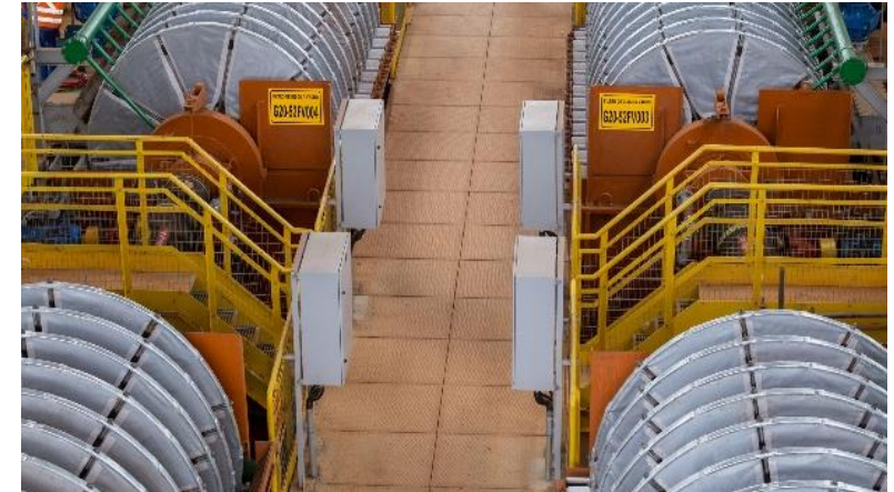
Samarco filtration plant
