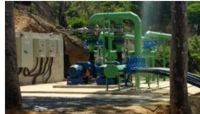
Santa Maria Pipeline in Colatina
