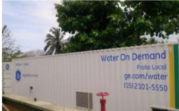
Mobile water treatment plants in Regência
