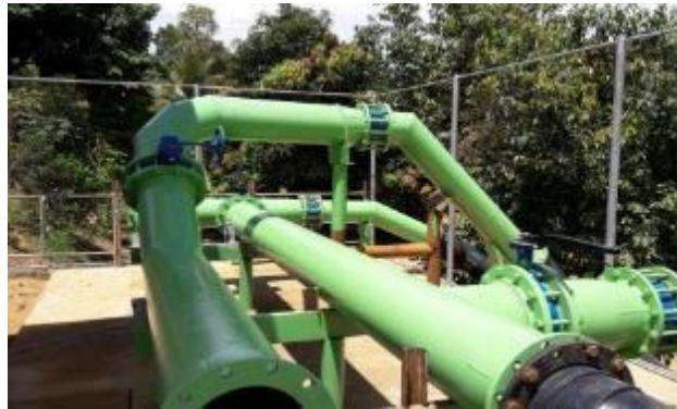
Pancas Pipeline in Colatina
