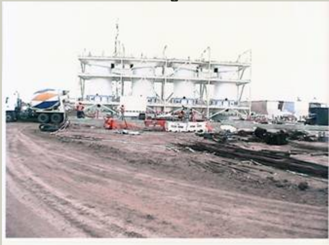
Ultra-fines microcell tanks
